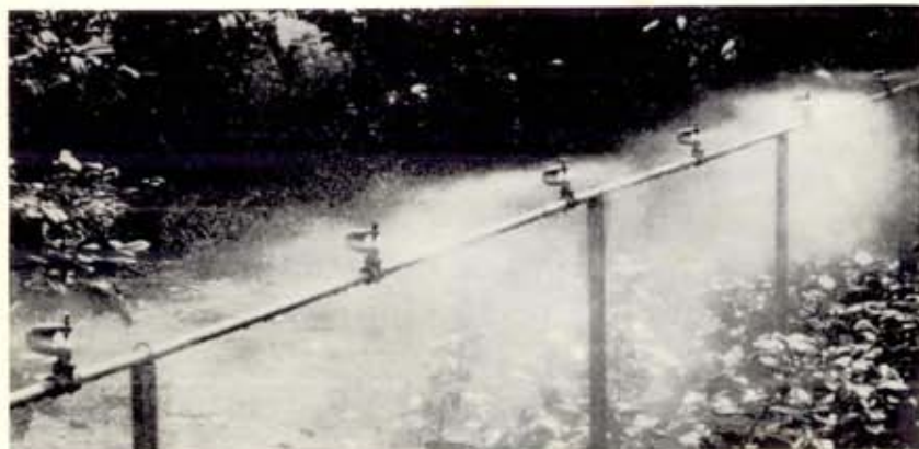
Typical Installation of Mister Bs in Series
